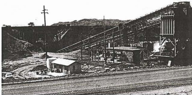
Truck Dump Hoppers and Conveyors One and Two Feeding Surge Hoppers
